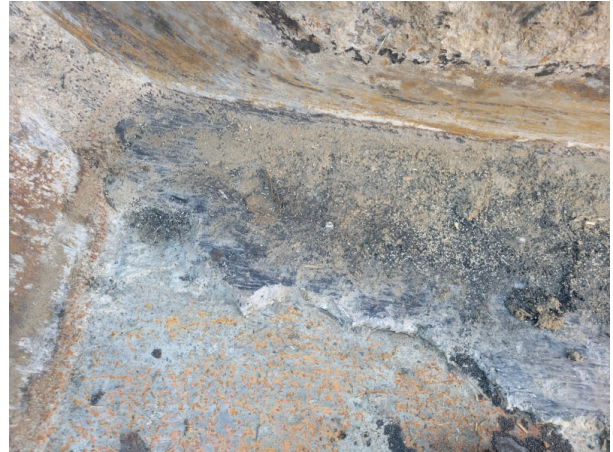
(Photo 4) Floor Seam
