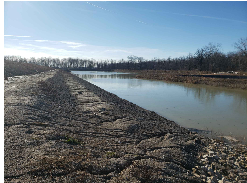
20 SURFACE WATER POND D Fig 4A
