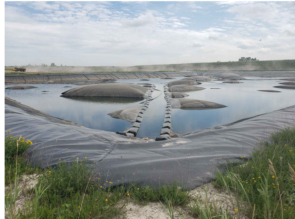
12 PONDED WATER ON EAST LEACHATE POND COVER Fig 4A
