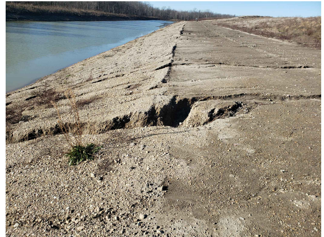
4 SOUTH ACCESS ROAD EROSION CHANNEL Fig 3A
