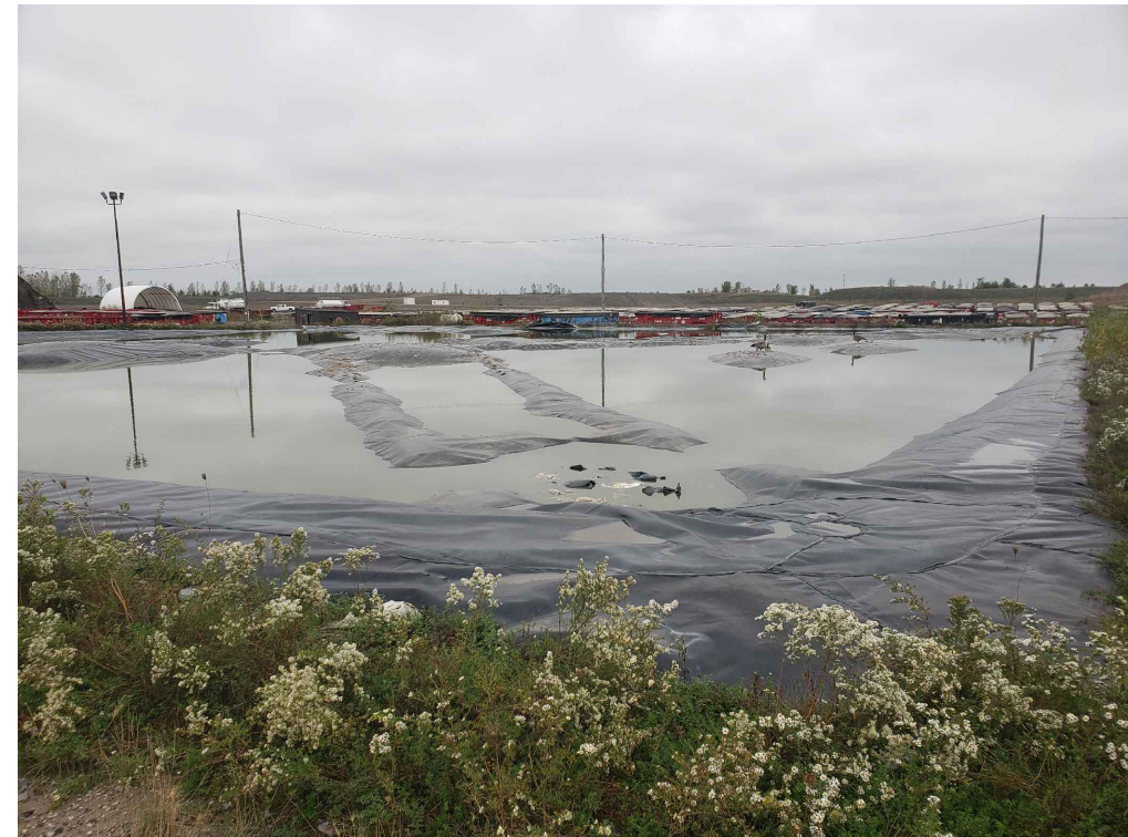
12 PONDED WATER ON WEST LEACHATE POND COVER Fig 4A
