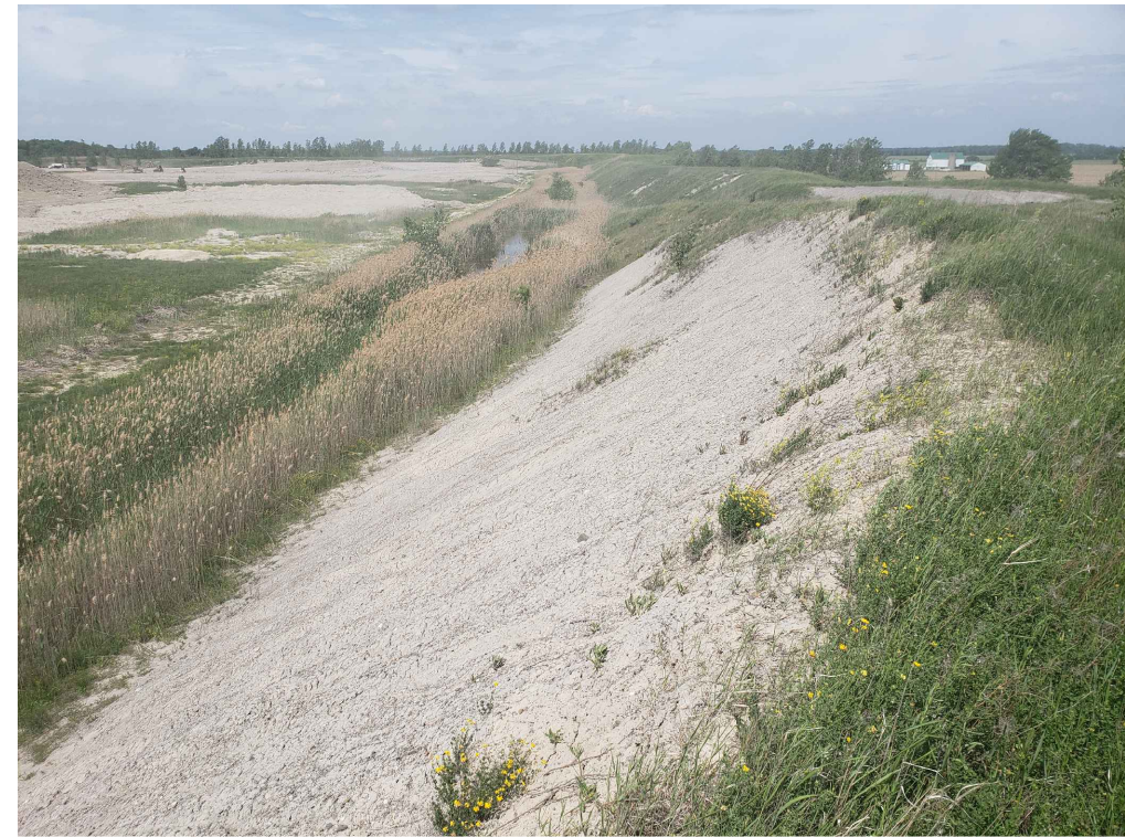
10 EROSION CHANNELS ALONG NORTH PERIMETER BERM Fig 4A
