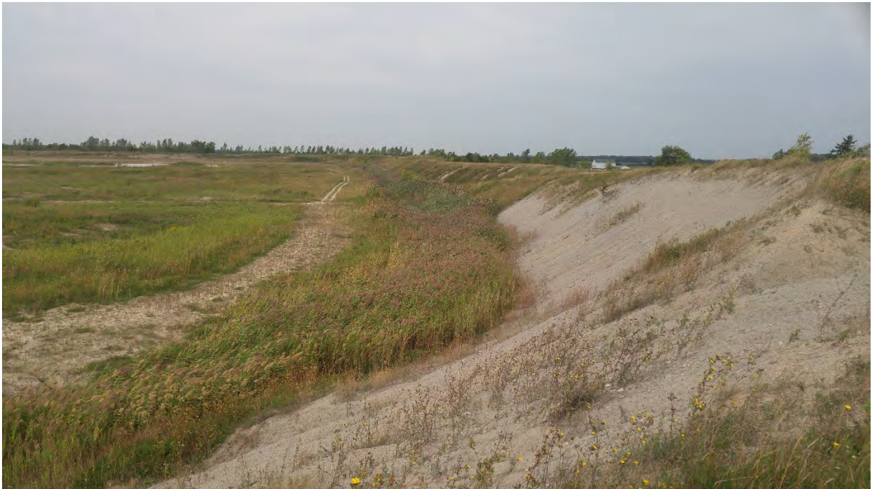
Photo 6 - North ditch, surface water blockage
