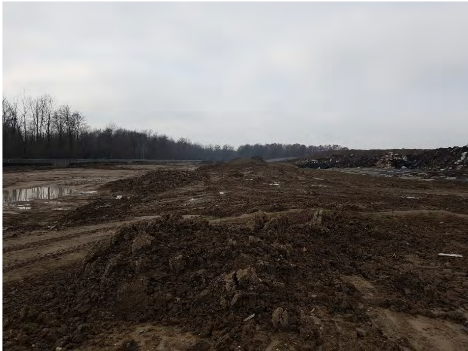
Photo 14 – Sitting water south of cell 19-1 and 19-2
