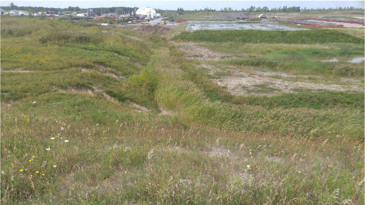
Photo 7 - Original Landfill Area, southeast ditch, partial surface water blockage
