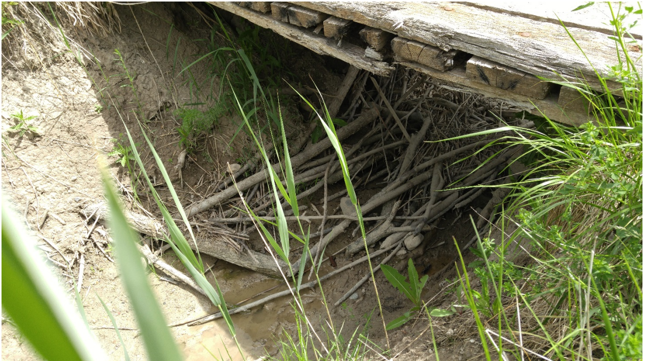
Photo 8 - South ditch, surface water blockage west of access bridge
