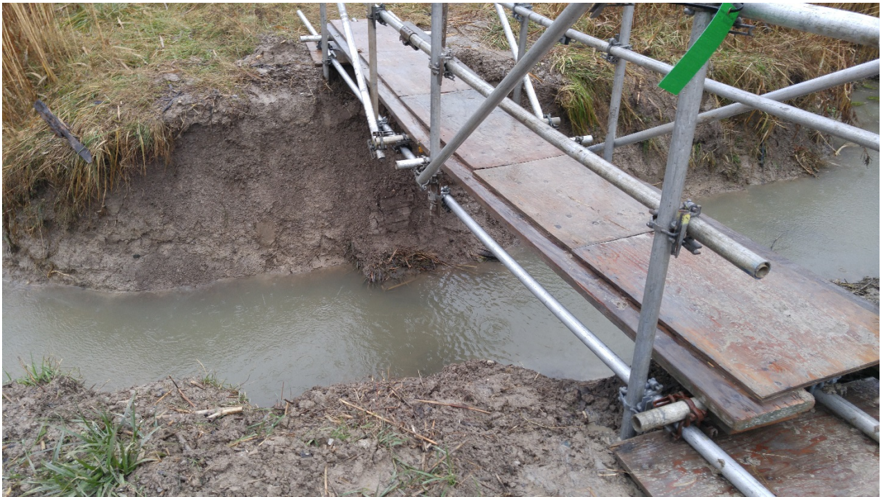
Photo 9 - South ditch, surface water blockage removed
