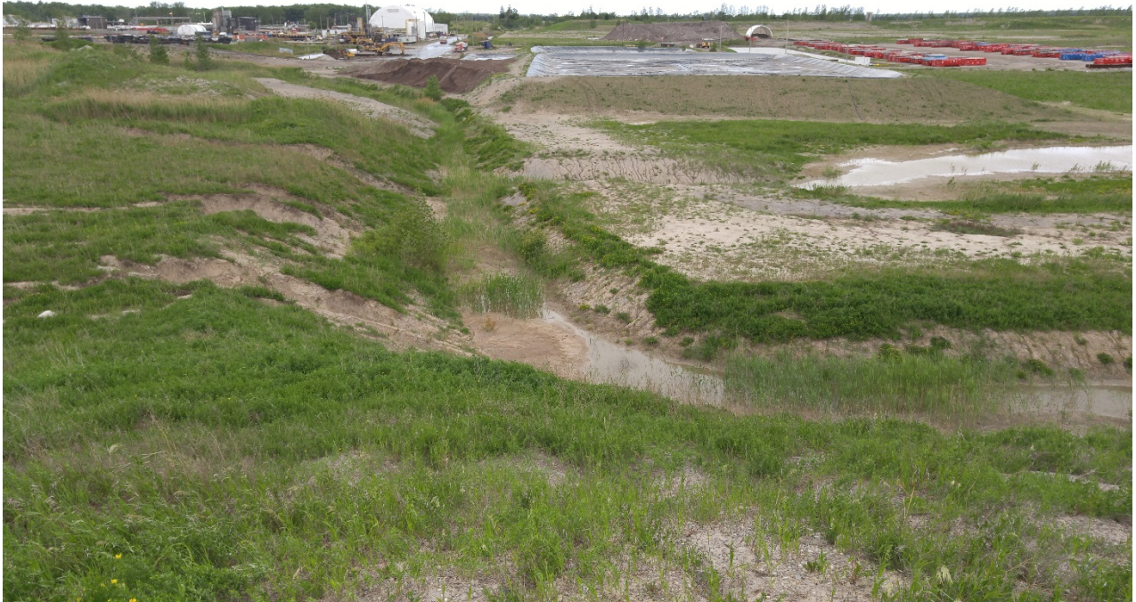
Photo 7 - North landfill area, southeast ditch, partial surface water blockage
