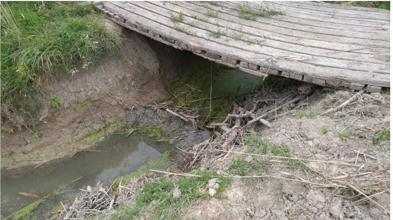
Photo 8 - South ditch, surface water blockage east of access bridge
