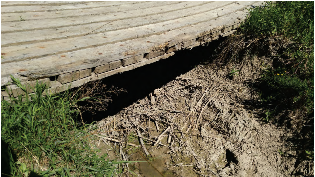
Photo 7 - South ditch, surface water blockage west of access bridge
