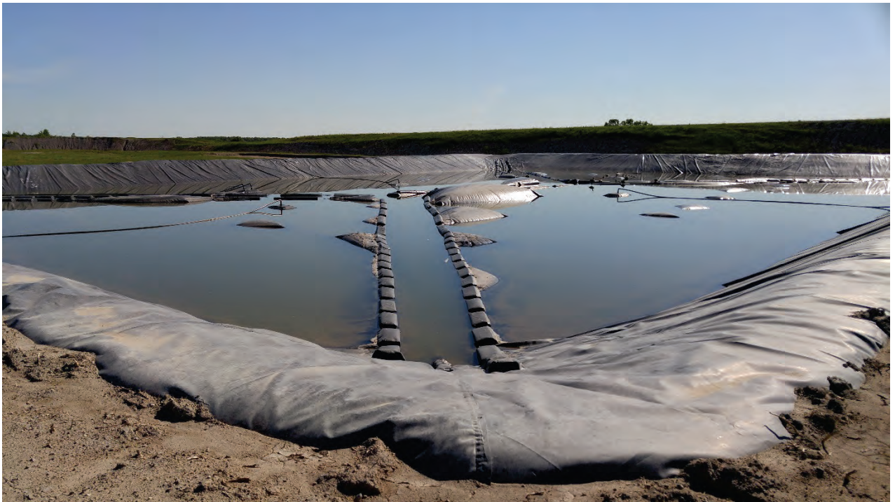
Photo 17 - New Leachate Reservoir
