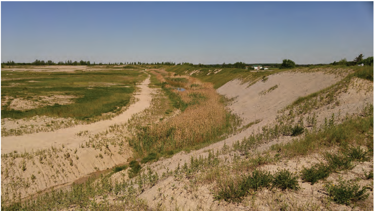
Photo 5 - North ditch, surface water blockage
