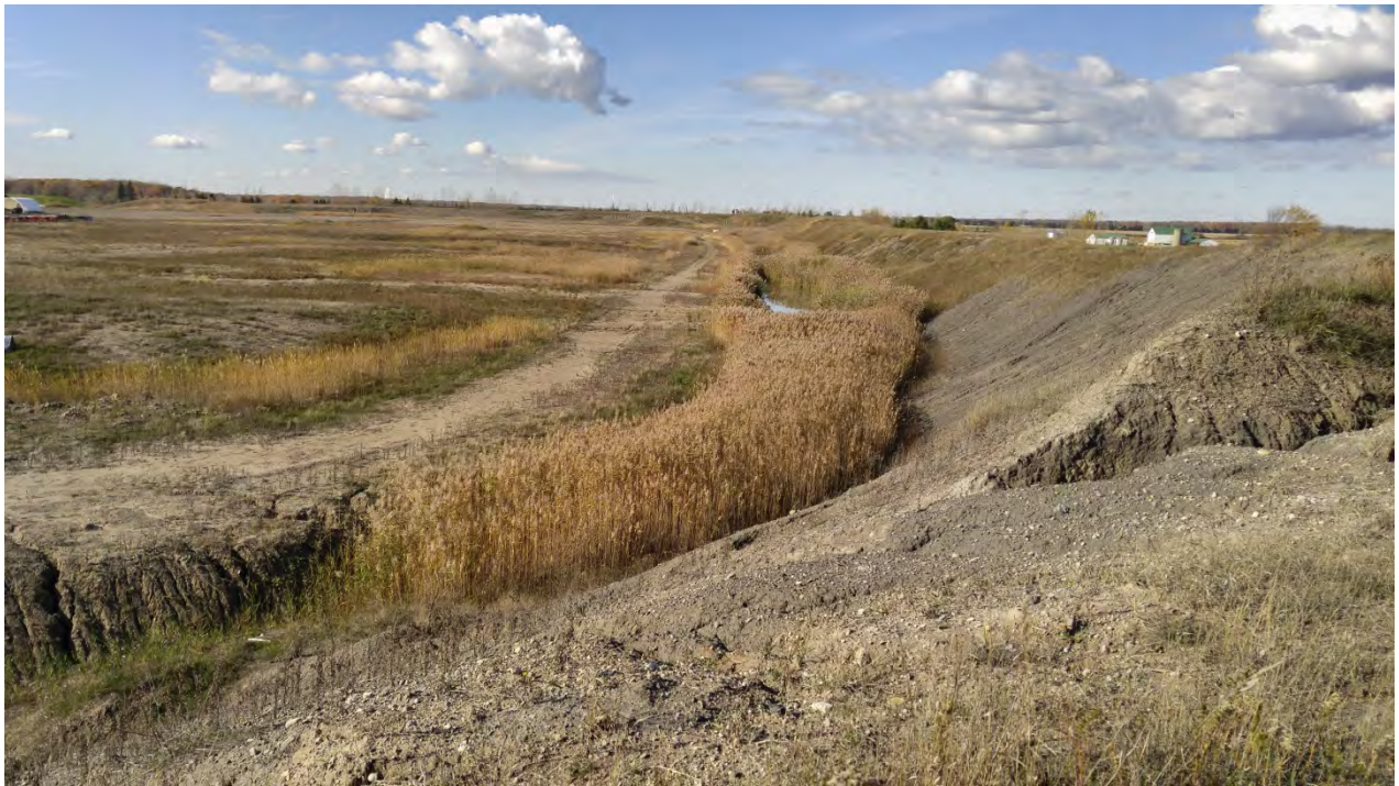
Photo 5 - North ditch, surface water blockage
