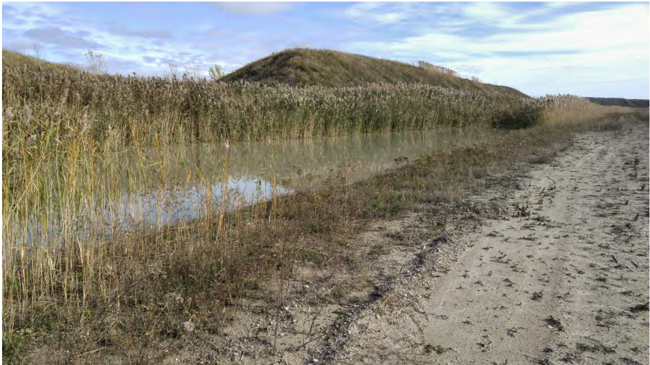
Photo 4 - High water levels in central portion of north perimeter ditch
