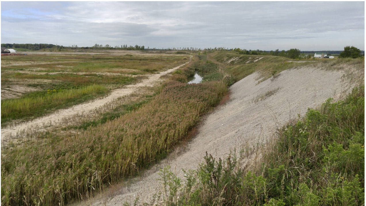
Photo 5 - North ditch, surface water blockage
