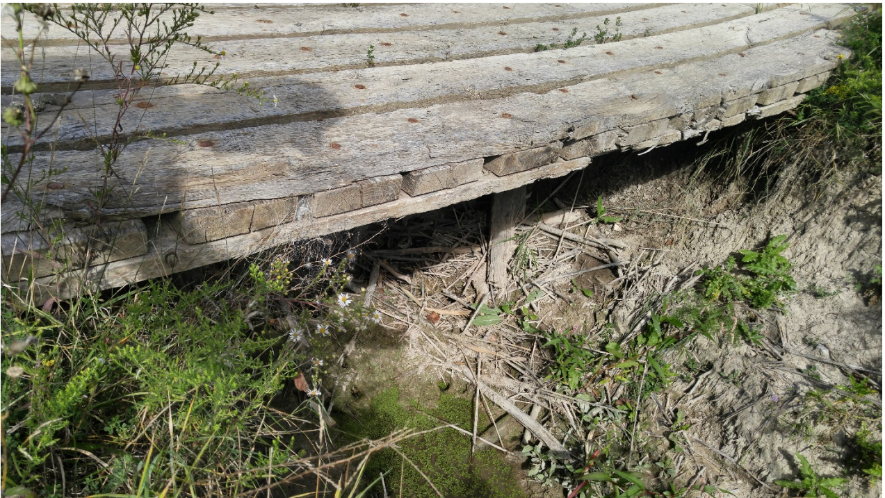
Photo 7 - South ditch, surface water blockage west of access bridge
